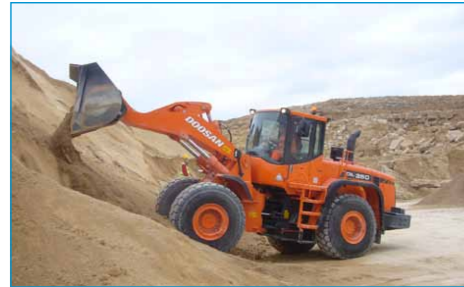
The DL350 on its 'first drive' at Johnson Quarry Group's limestone quarry in Creeton, Lincolnshire.
